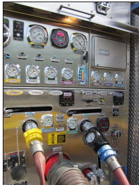
Figure 31: The pump discharge pressure was raised to 100 psi and water transfer operations were started. Subsequent tests were completed with pump discharge pressures set to 125 psi and 150 psi.
