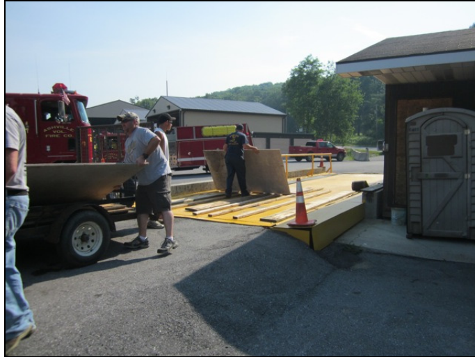
Figure 20: Crews work to build a wooden platform on the scale so that the 3,000-gallon collection tank rests entirely on the scale and does not touch the side rails.
