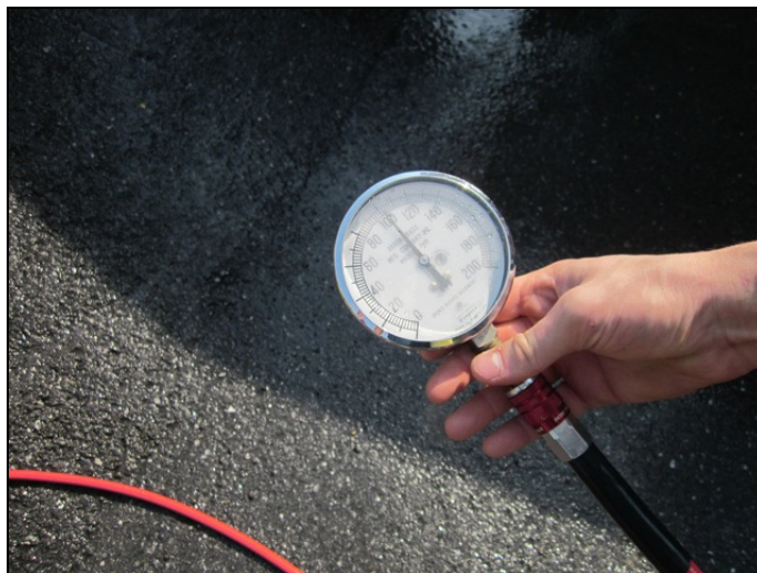
Figure 33: A pressure reading was recorded on the in-line test gauge located at the jet siphon device's supply inlet.
