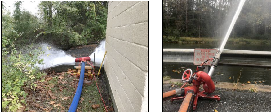
Figure 7: The Hose Monster was outfitted with a 2-1/2-inch orifice. The portable monitor was outfitted with an Akron flow test kit and 1-3/4-inch orifice.
